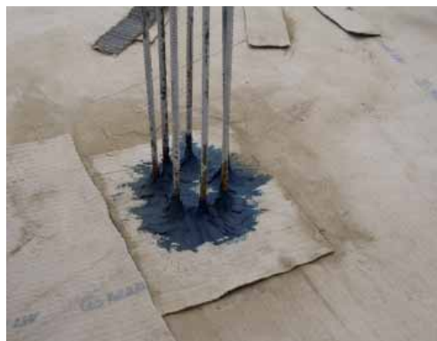
Fig. 3 - Sealing a piece of Mapeproof sheet around steel reinforcement rods with Mapeproof Mastic
